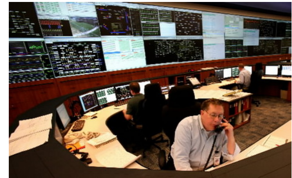
Transmission System Control Room
